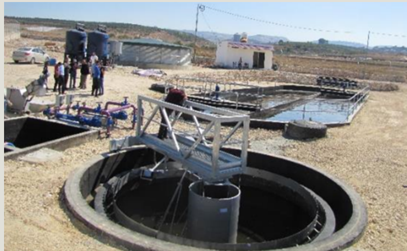
Wastewater Treatment Unit
